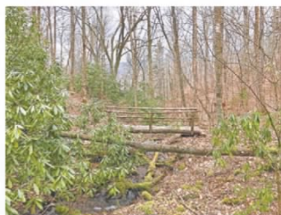
COURTESY OF CHRIS HIGHLAND Bridges may be built by people or provided by nature.
