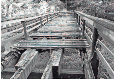
This broken bridge was under repair at the Botanical Gardens of Asheville. CHRIS HIGHLAND/COLUMNIST
